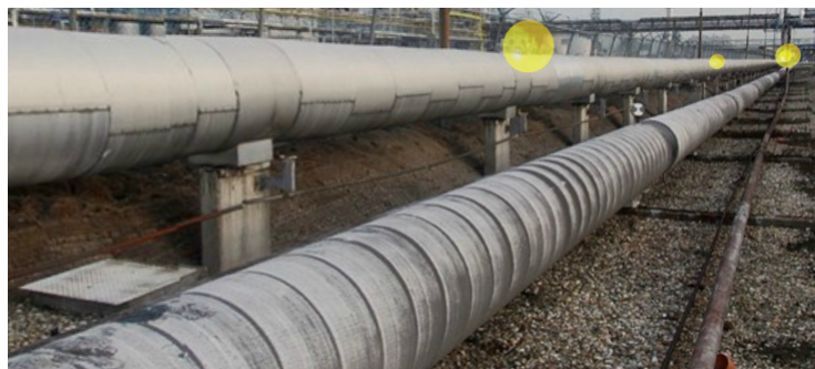
Figure 44: Pipelines stretching across multiple scans. This view is taken from one scanner, the yellow spheres are the positions of nearby scanners.
