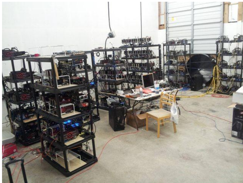
Figure 3. Photograph of a Bitcoin mining server farm. Source: http://25.media.tumblr.com/tumblr_m3sp4m5Oda1qfy0bho1_1280.jpg
