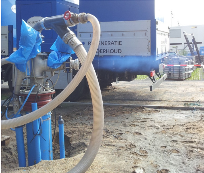
Fig. 24. Pressure release during the process of surging.
