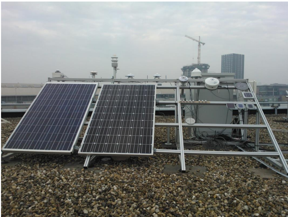
Figure 6 Picture of the test installation of EKO Instruments Europe, showing two crystalline solar panels on the left and the equipment to measure incident spectral irradiance on the right. The amorphous-silicon modules are not captured in this picture, but are located to the right side (source: EKO Instruments Europe).
