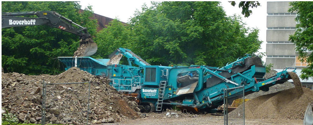
Figure 3.4 – Mobile crusher. On the left rubble is inserted in the crusher. In the middle ferrous-metals are separated from the rest of the stream. The output on the right is aggregates, which can be used to replace grind or sand in the production of stony building material.
