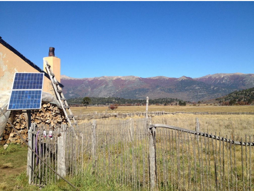
Figure 15: Photo Solar Panel
