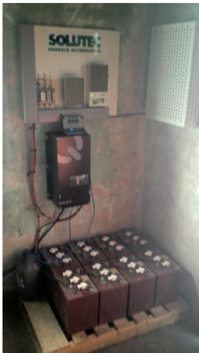
Figure 12: Batteries Wind Turbine
