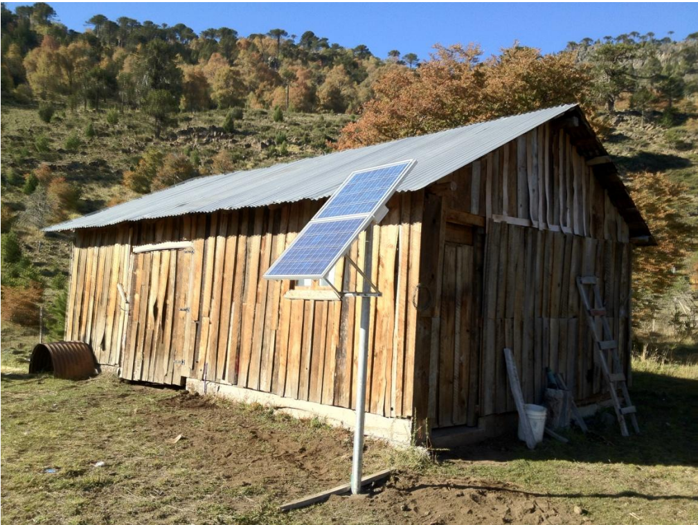
Figure 14: Photo Solar Panel
