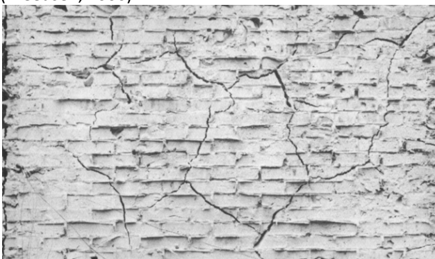
figure 4.1.7 cracks in UF-foam visible after the outer wall is removed (Meeusen, 2006).
