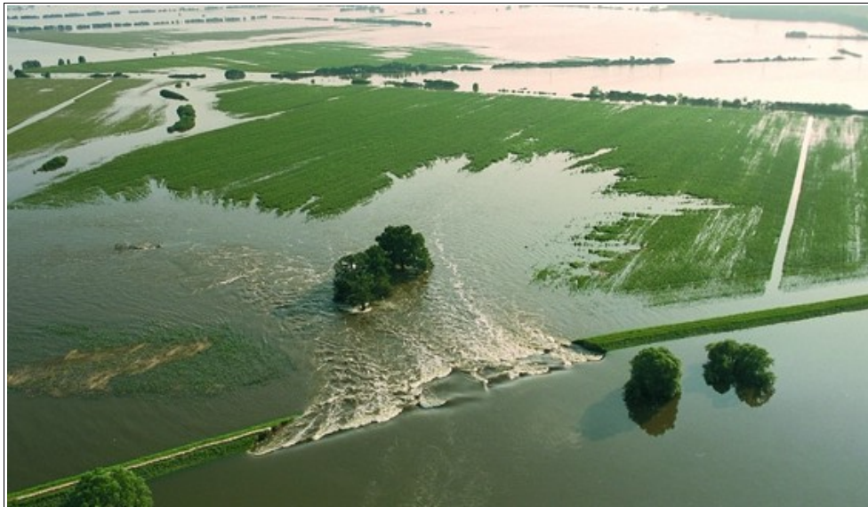
A dike has collapsed (source: MKULNV, 2011b, p. 14)
