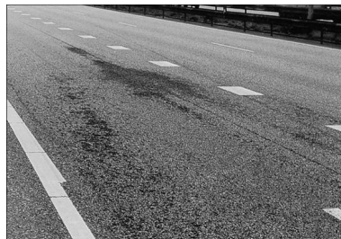
Figure 1.4: Severe raveling of a road
